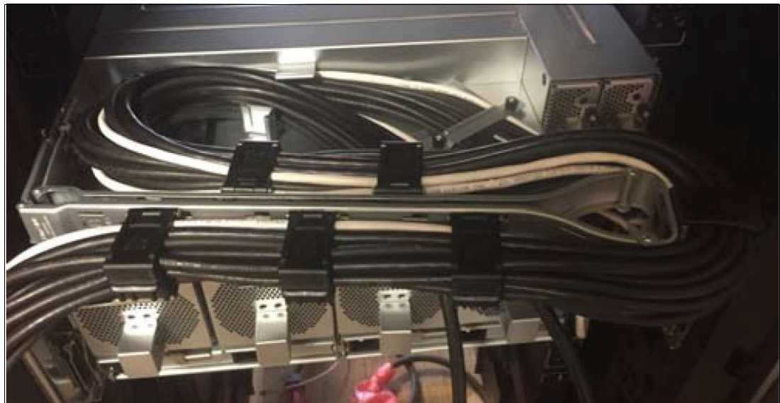
Figure 3-19 Cable management arms and cabling
